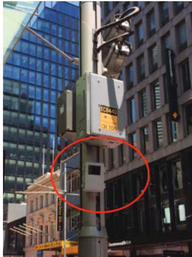
An example of a camera used for data capture mounted on a light pole
